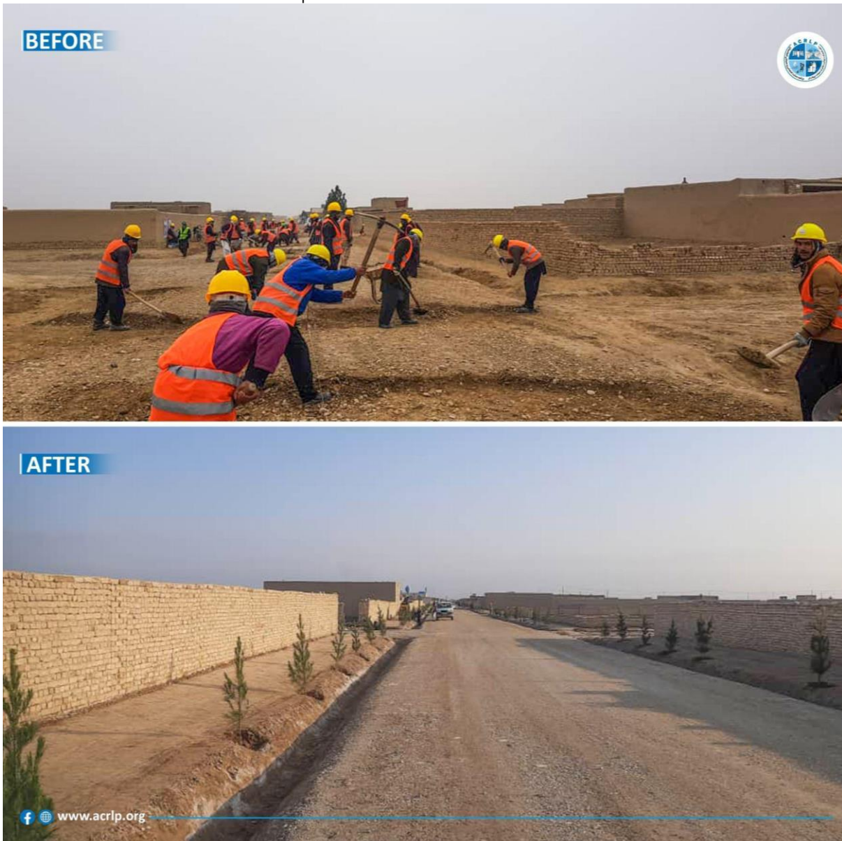
Photo: Before and after condition of gravel surface road in District 9 of Mazar-e- Sharif on February 15, 2023
